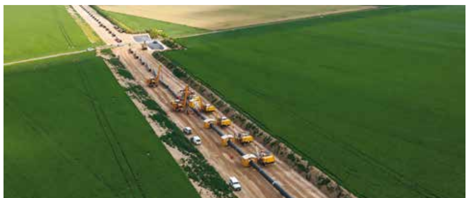
Max Streicher GmbH & Co. is laying 51.7 km of 48 inch, DN 1200 gas pipeline on behalf of GRTgaz as part of the Haute de France II project.
